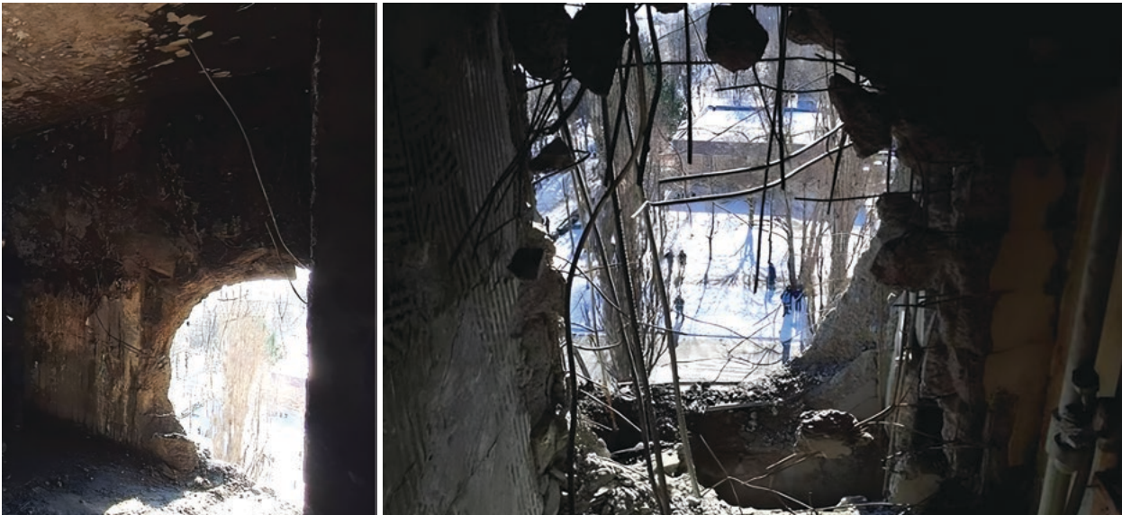
Fig. 4 | The image of opening in the wall panel of the 8th floor at the UAV impact place
